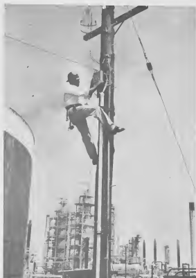
FRAMED by the refinery and a clear Caribbean sky, H. Semelcer of the telephone exchange tests telephone lines at a terminal.
